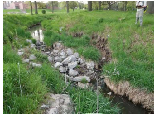
Figure 7-7: Failing Grade Control
